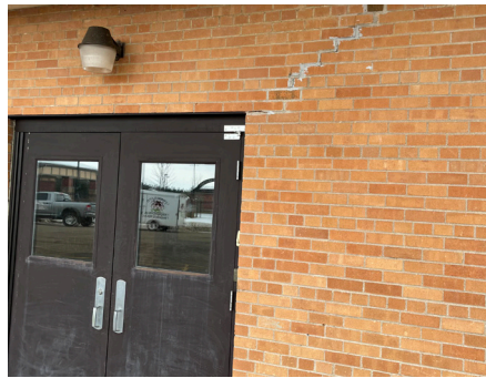
Exterior Envelope & Structural Issues
