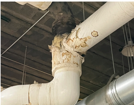
Failing Pipes with Asbestos
