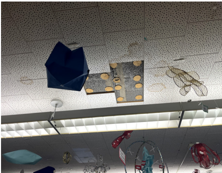
Failing Interior Finishes
