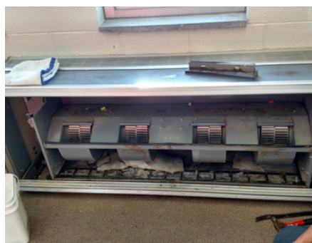
Failing HVAC Systems
